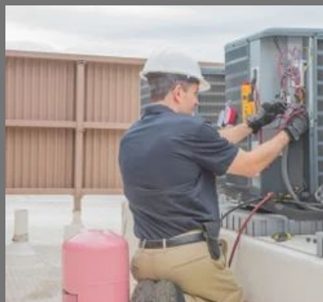
Regular Maintenance Services
