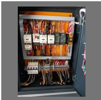
Chiller Electrical Panel Wiring Service
