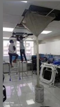
Industrial Air Conditioning Maintenance Service
