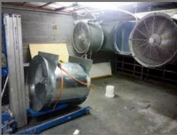
Industrial Cooling System Services
