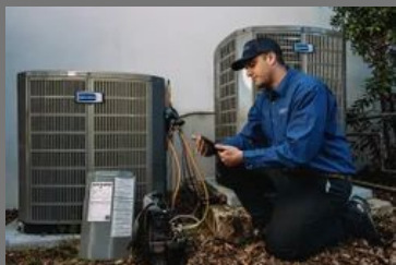
HVAC System Maintenance Services
